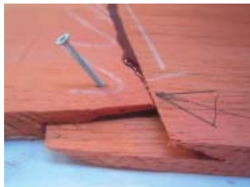
Slim crosshead screws, available from most builders' merchants, locate the joint and...
