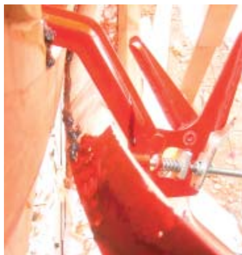
Looking down on the joint with the Sika marine mastic at the top of the picture and the RS12 resorcinol adhesive lower down.
